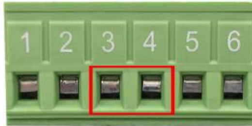
Figure 2-16: 6-Pin Terminal Block Fault Alarm contact
